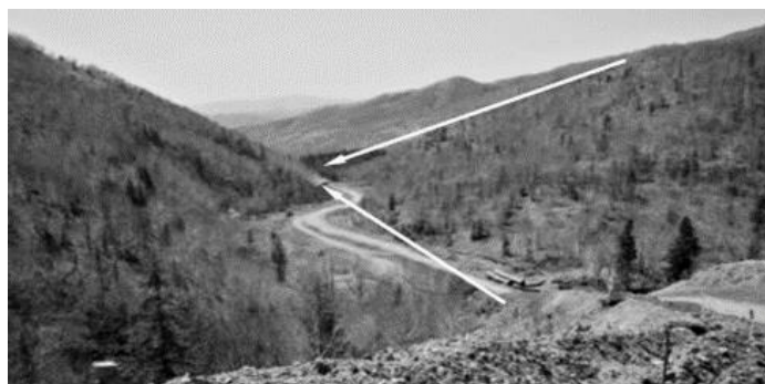
Figure 1 – Laying of the pipeline in the mudflow of the Pulka River (Kazakov, 2008)
